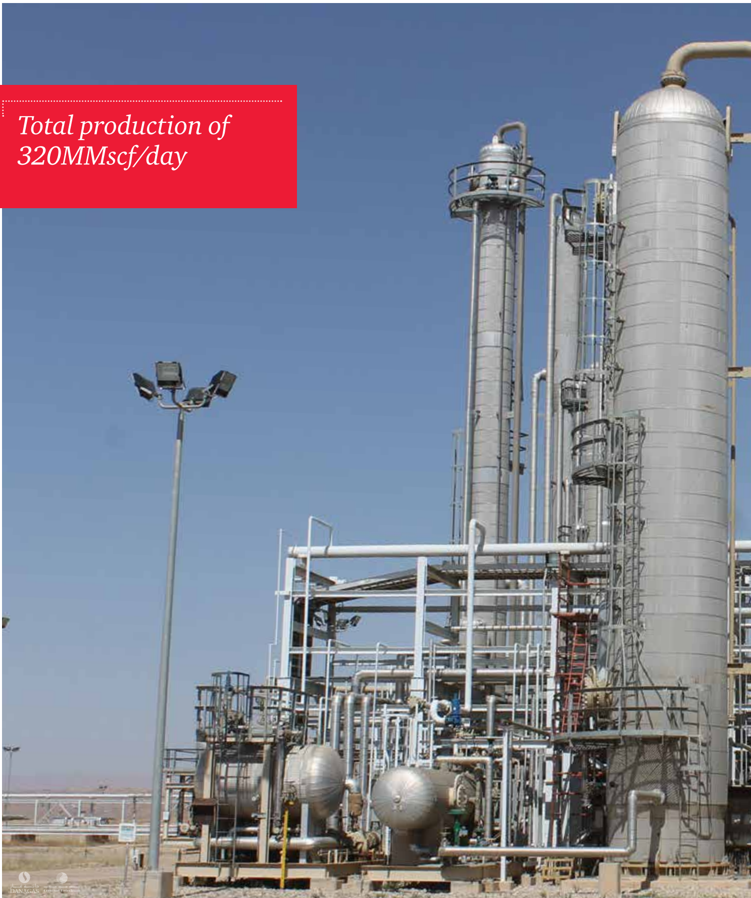
DGCP's Amine unit, LPG Plant
