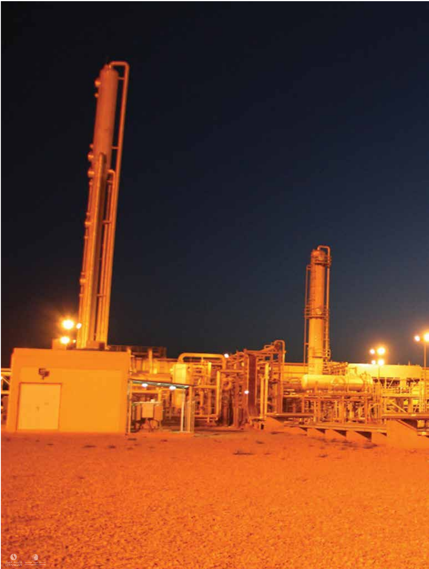
DGCP Khormor Gas Plant – providing electricity to power KRI's industry
